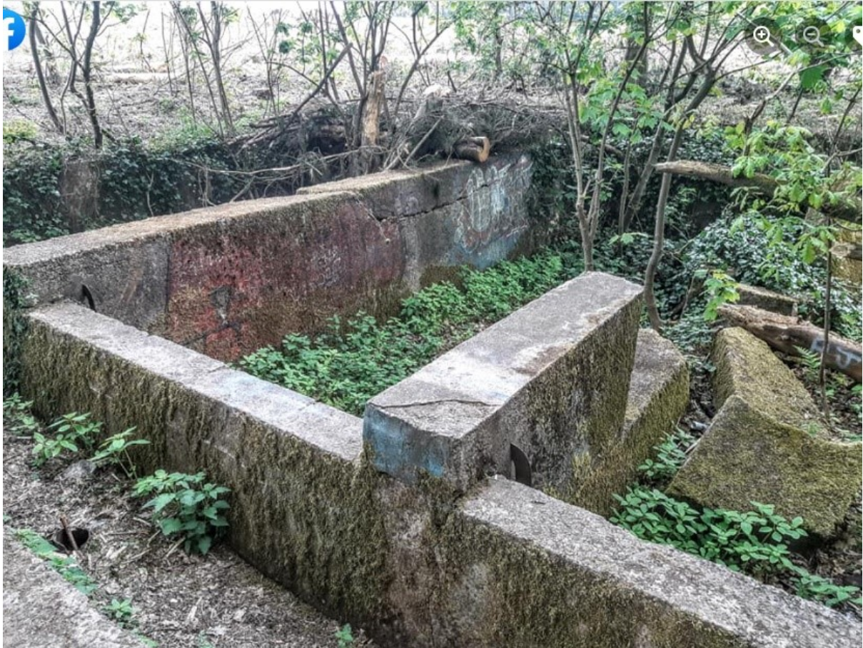
Figure 40 The remains of the Sewage works photographed by Tim Priestley (Priestley, WW1 Clipstone Camp, 2020)
